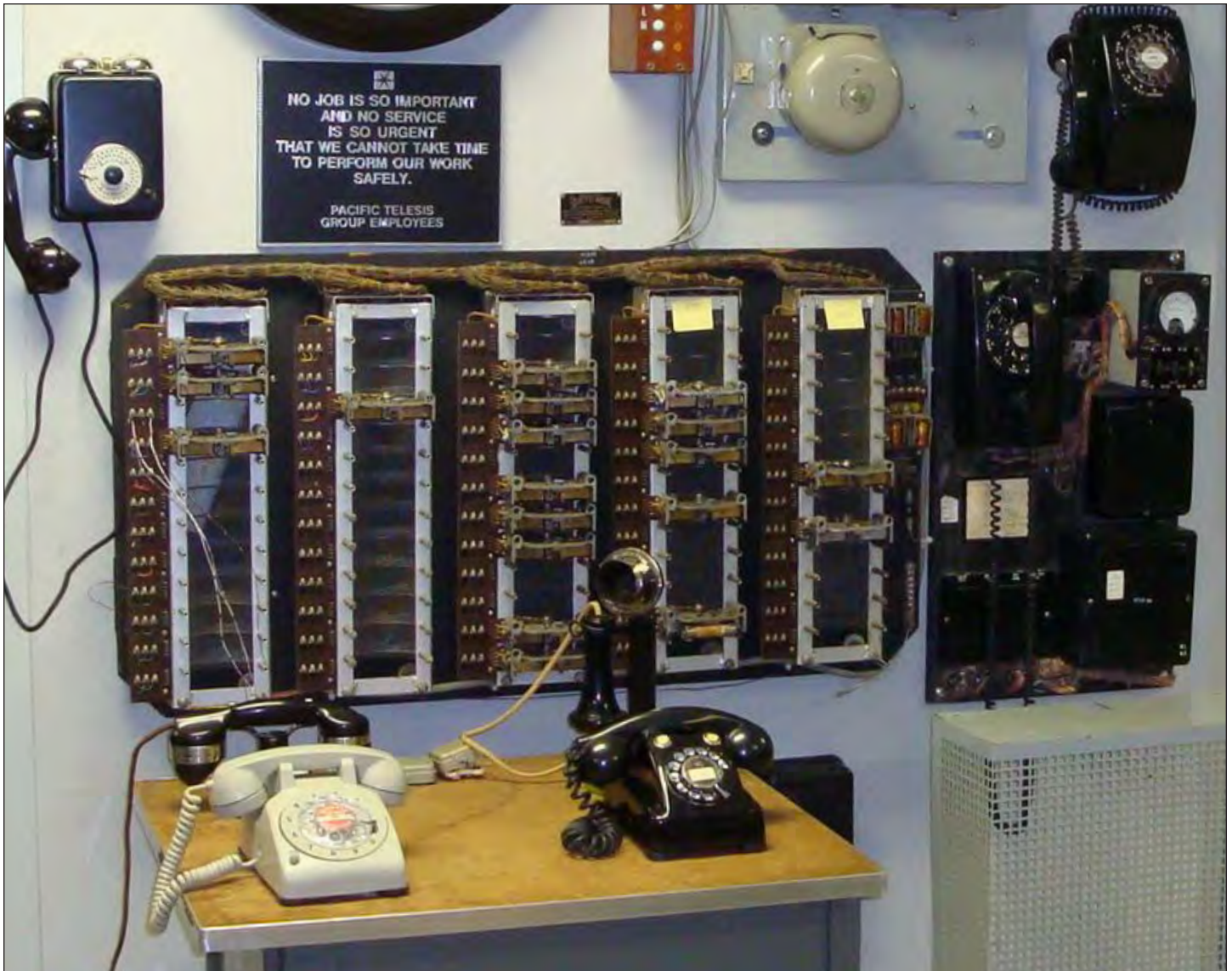
A Kellogg Select-O-Phone switch, refurbished, rebuilt, and installed by Mike Neale at the JKL Museum.
